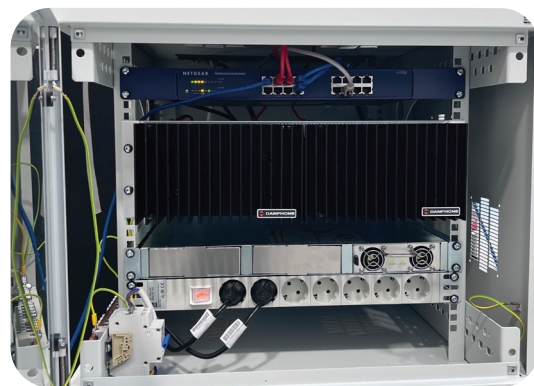
Danphone VHF Transceivers operating in the marine VHF band mounted in rack.
